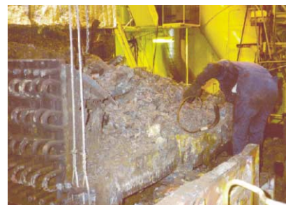
Melt down as a result of soot fire.
