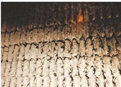
Cleaning of heating surface highly overdue.
