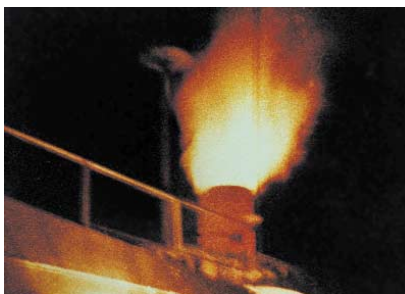
Soot fire raging from the stack.
